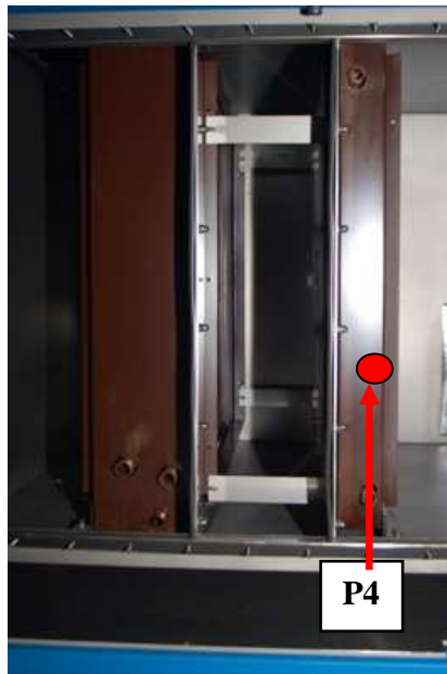
Figure 6 Pressure probe between the heater and the cooler
