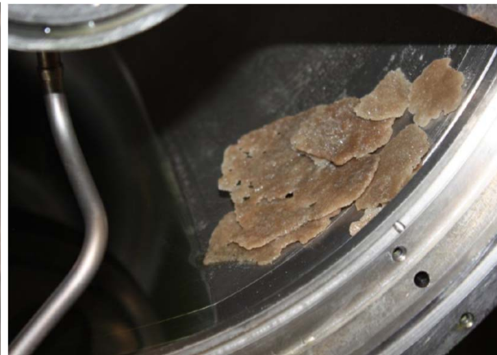
Scaling in evaporator
