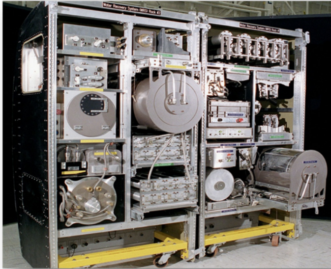
Racks for the ISS water recovery system (Carter et al. 2011)
