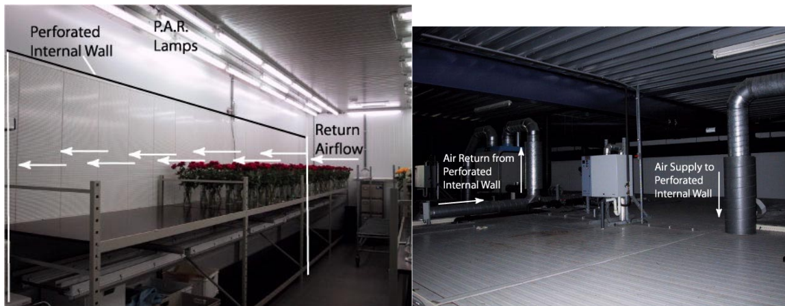
Figure 6.5: Inside and outside photos of growth chamber with displacement ventilation system: Left: Internal perforated supply and return walls (return only shown), Right: External overhead ducting
