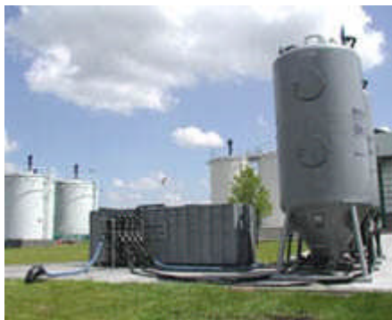
Figure 35: Industrial aerated activated carbon filter
