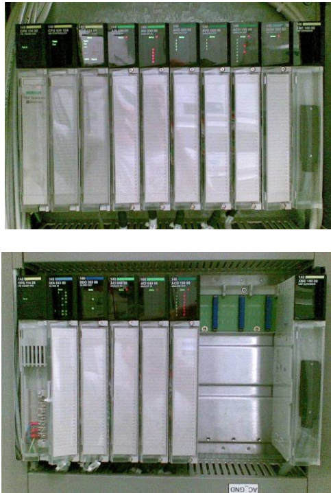
Figure 6: PLC assembly on backplanes
