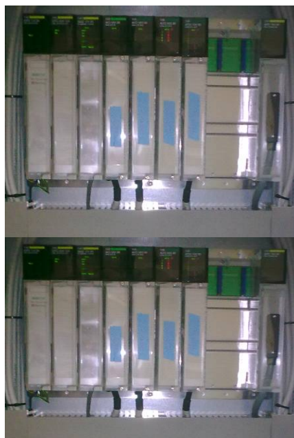
Figure 7: PLC assembly on backplanes
