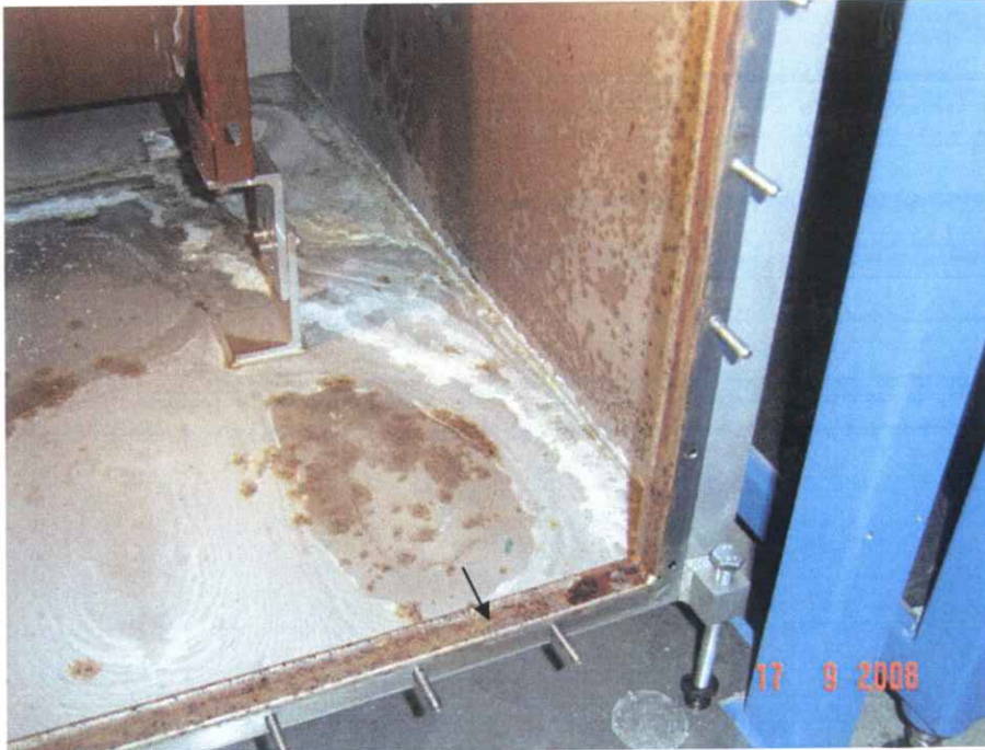
Figure 1: The lower air recirculation chamber floor. Samples were taken of the rust coloured deposits on the floor and wall and of the white coloured deposits on the floor. The open circuit potential was measured in the corroded area on top of the frame and the clean area on the front of the frame.
