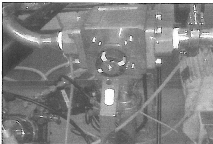
Fig. 8. Position of the three-way valve H3V_1001_01 for emptying the WPU to the drain system.
