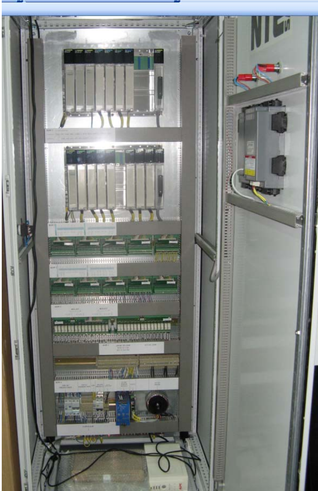
Figure 5-23 HPC Control Cabinet assembled
